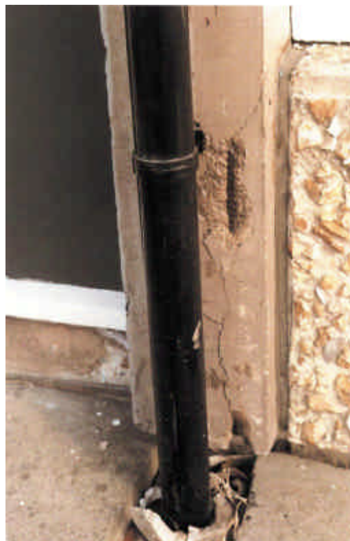
Figure 12 Shepard Spacemaker LPS building with extensive cracking and spalling in exposed ends of cross walls
